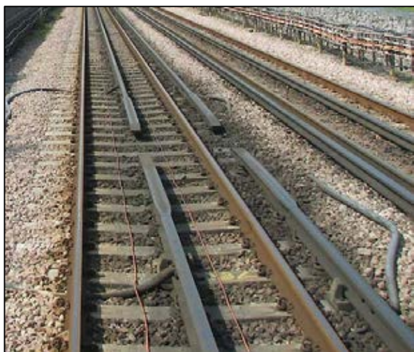
Figure 29: Photo of part of London Underground track (Jubilee Line) showing conductor rails with a gap as provided at a substation. Photo: Richard Griffin.
