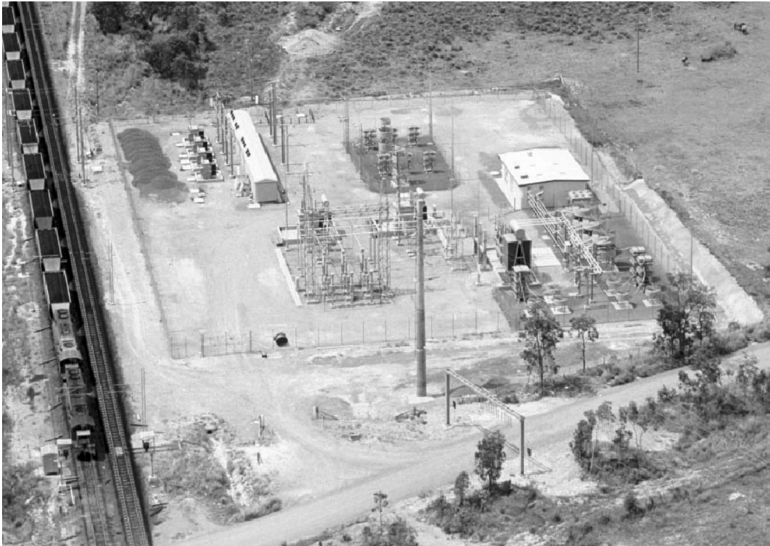
Fig. 5.2: Aerial view of the SVC installation yard along side the rail-track [58]
