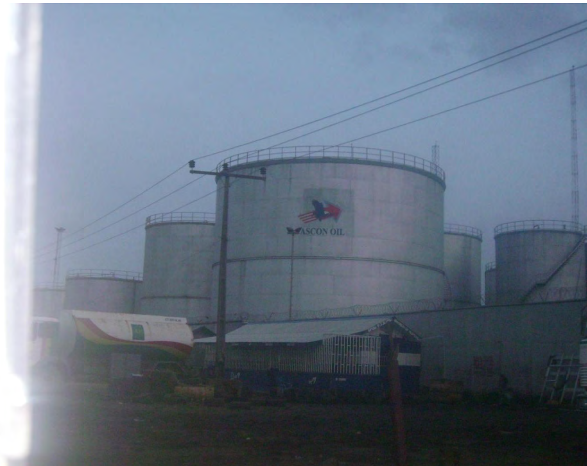
Figure 6.5: Tank Farm in Apapa Lagos State
