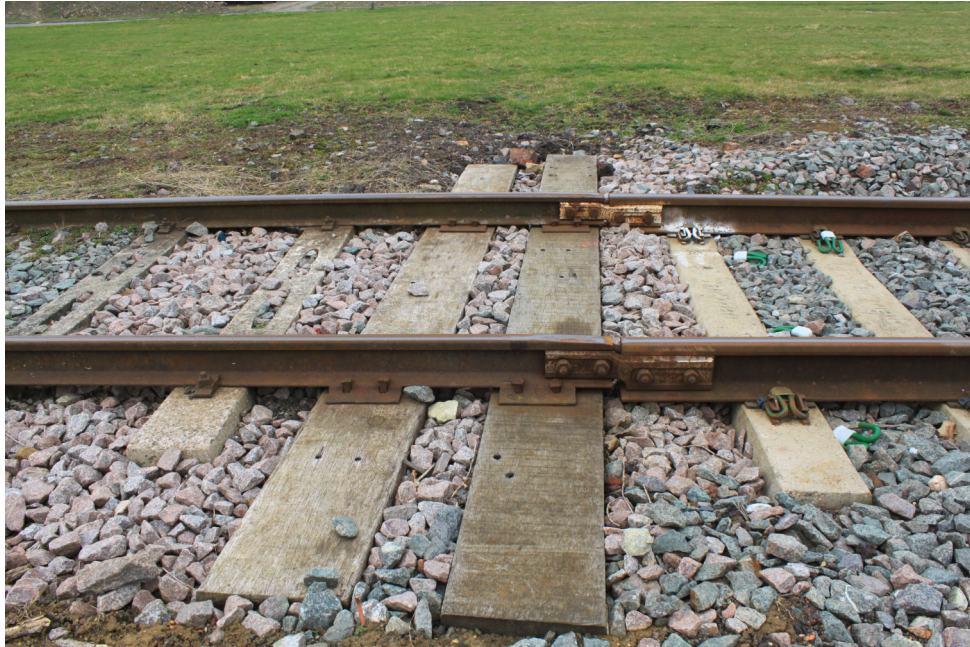
Figure 7.14: Compromise joint before Site 2
