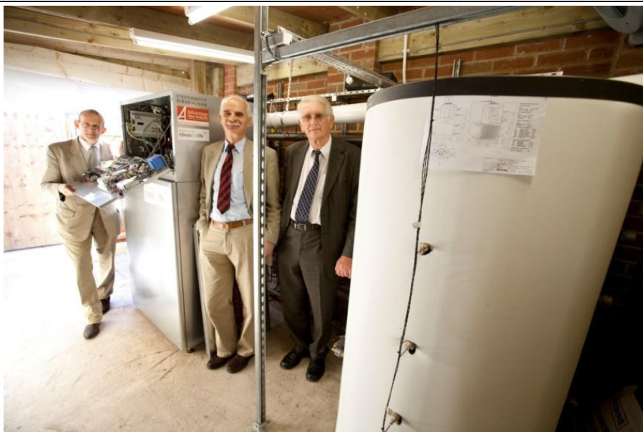
Figure 2.5: The Baxi Beta 1.5 fuel cell system and a 600 litre Gledhill heat store that were installed into an outdoor enclosure at a demonstration house in the UK. The hot water tank measures approximately 1 by 1.75 metres, and weighs nearly three quarters of a tonne when full.
