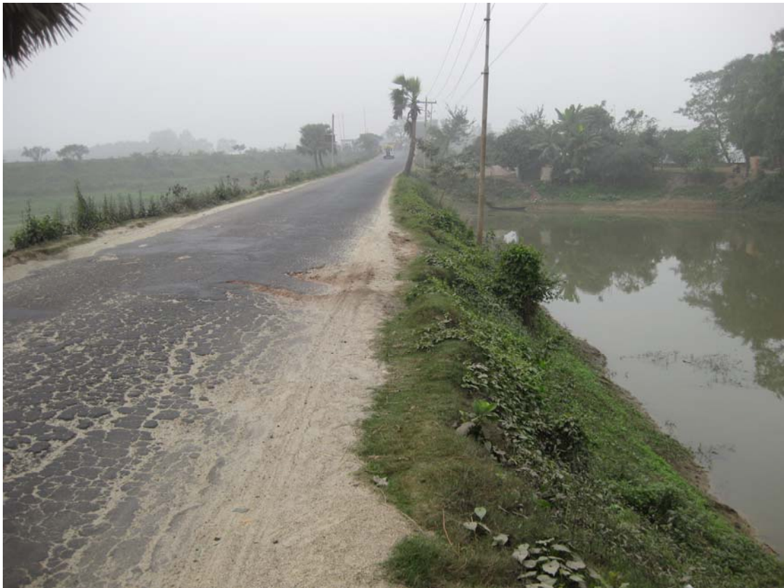
Figure 4 Settlement and slope failure of Kaliganj-Ghorashal Road
