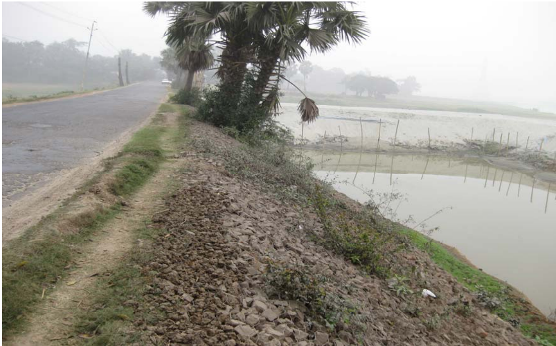
Figure 1: Slope failure of Kaliganj – Ghorashal Road.
