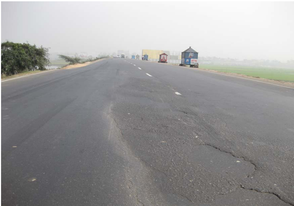
Figure 2: Slope failure and differential settlement of Tongi-Ashulia Road
