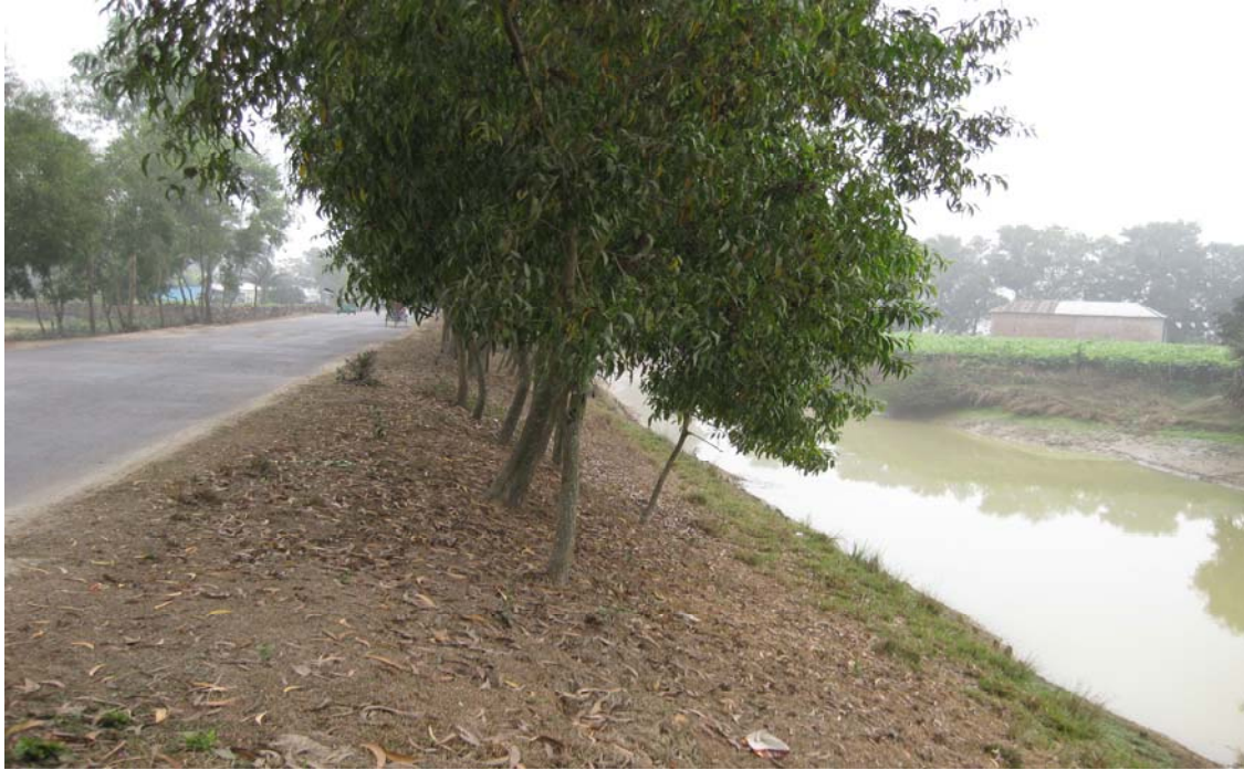
Figure 3: Slope-failure due to cutting at the toe of embankment of Dhaka bypass
