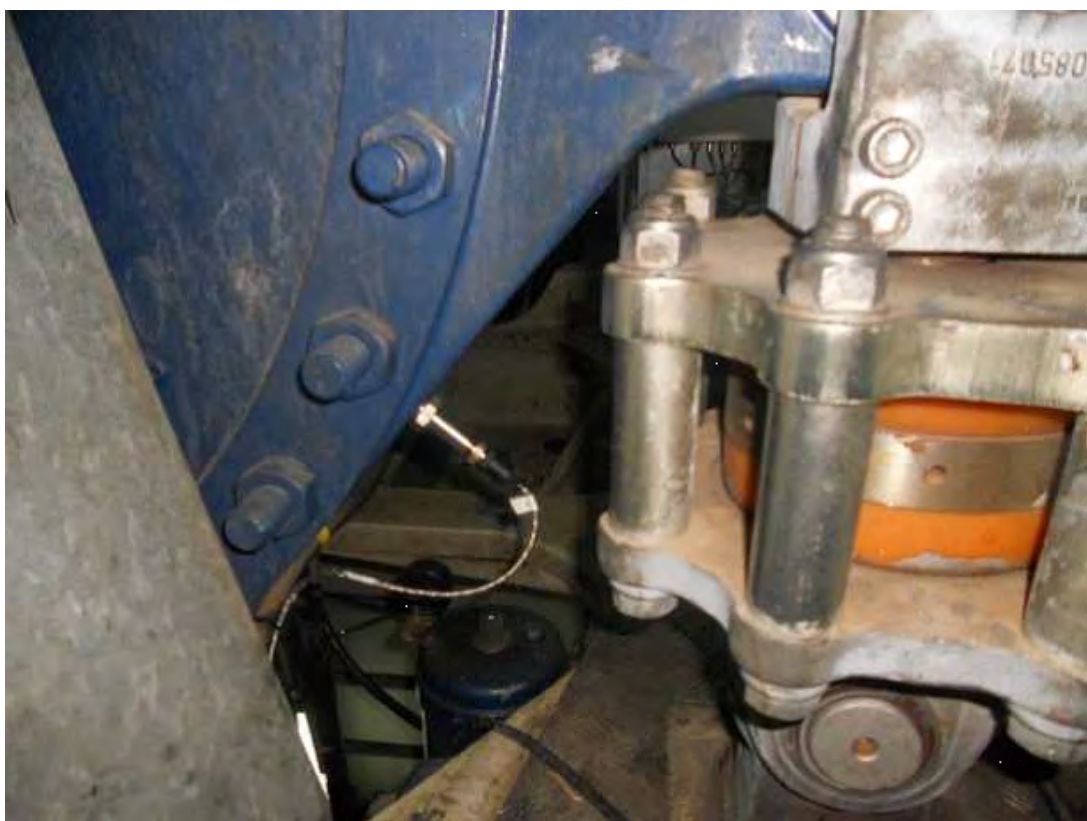
Figure 6.22: Installed sensor on the wind turbine M2; top: Generator Drive End Radial and Axial sensors, bottom: Planetary Radial Sensor (Photographs are courtesy of Ingeteam).
