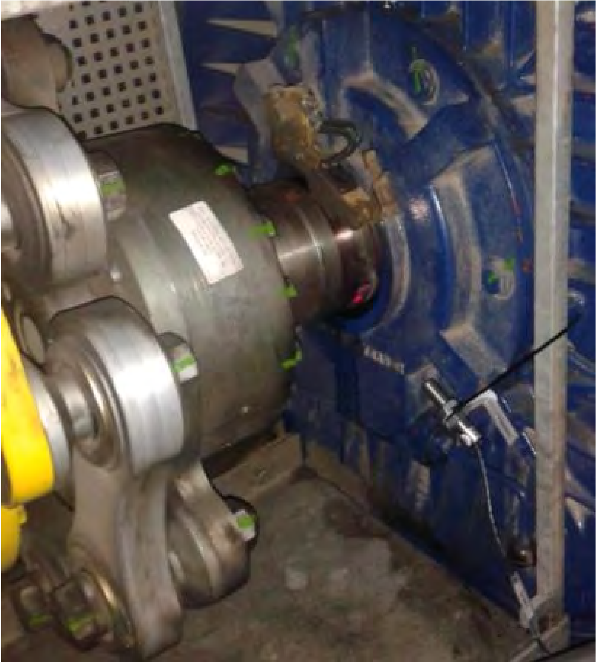
Figure 6.6: The tachometer installed on the high-speed shaft going to the generator (Photograph is courtesy of Indra).
