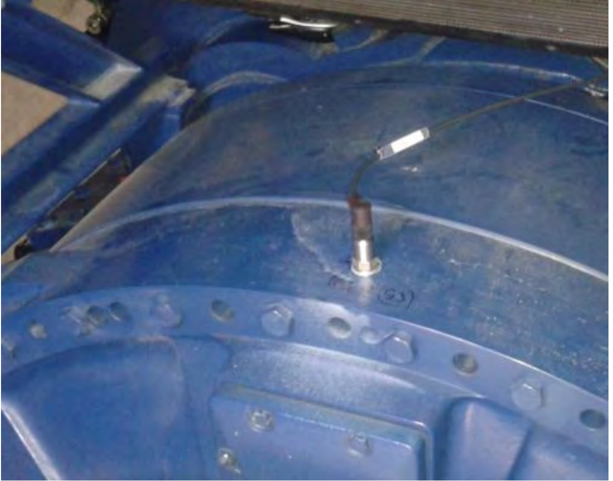
Figure 6.5: The L3 (MEV) sensor located on top of the planetary gearbox (Photograph is courtesy of Indra).
