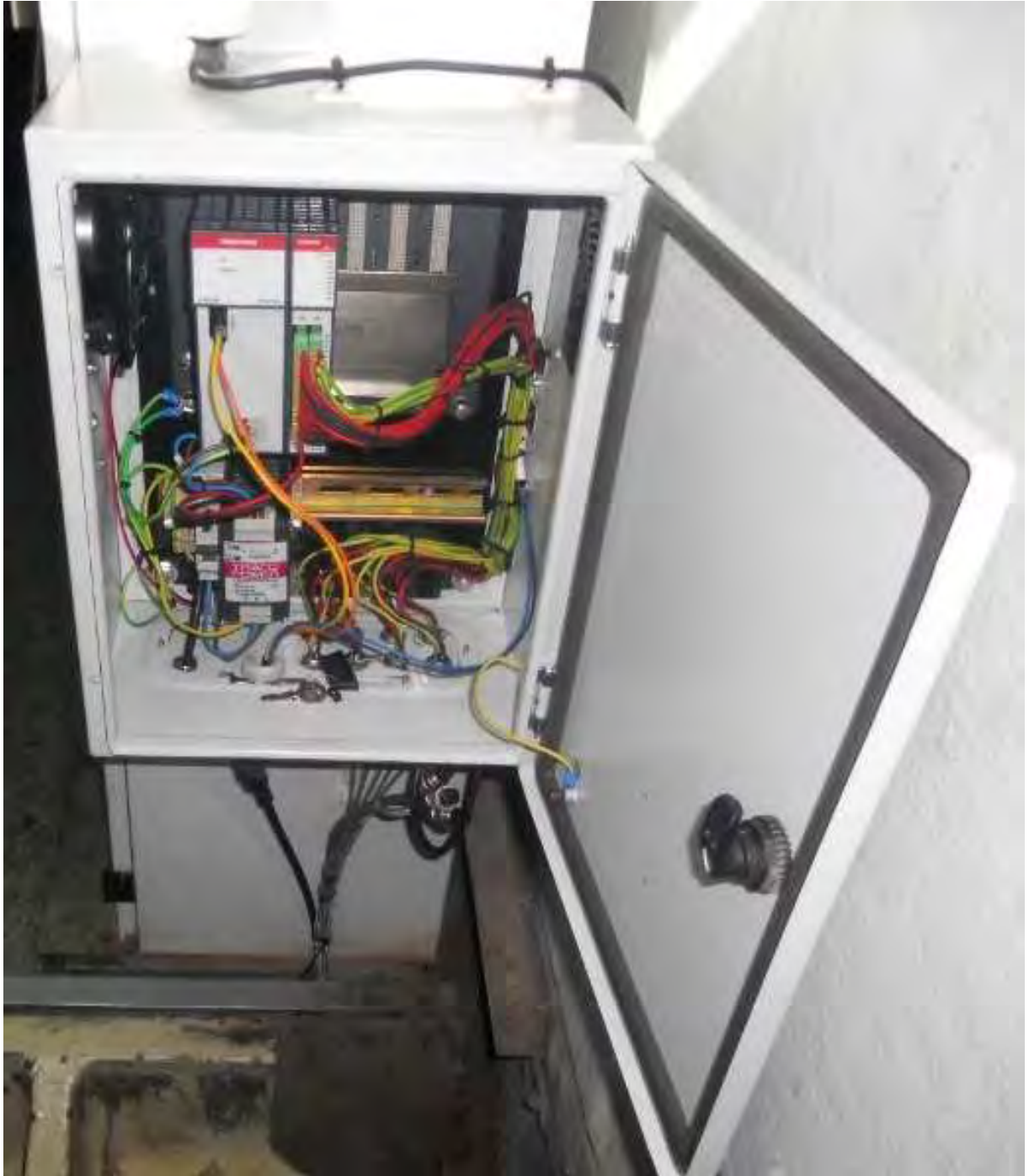
Figure 6.23: Ingesys CMS system located in nacelle containing Data acquisition, communication and power unit (Photograph is courtesy of Ingeteam).
