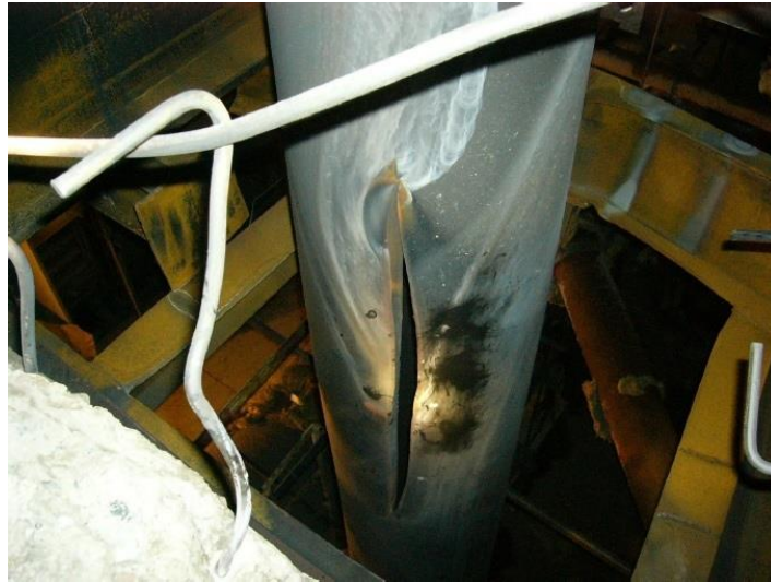
Figure 4-1: Grade 91 main steam pipe rupture at Huadian Datong Power Plant, China [194]
