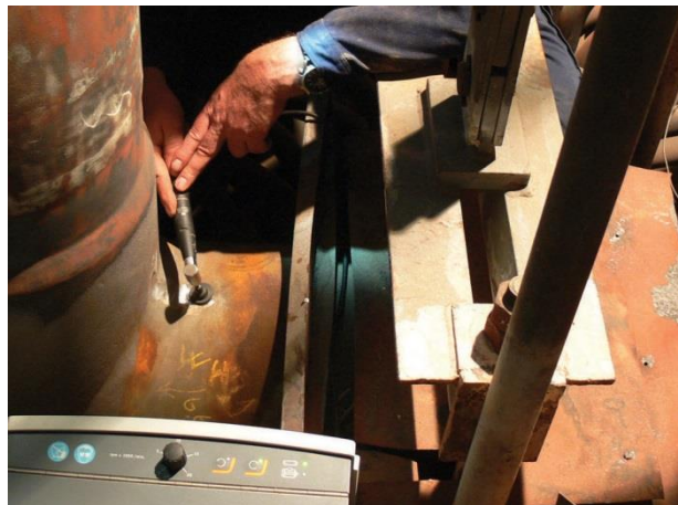
Figure 3-6: Example of TransPol-5 hand grinder being used to prepare a local surface area on a boiler component; typically used to prepare surfaces for surface replication, as it is capable of producing a mirror-like surface finish [191]
