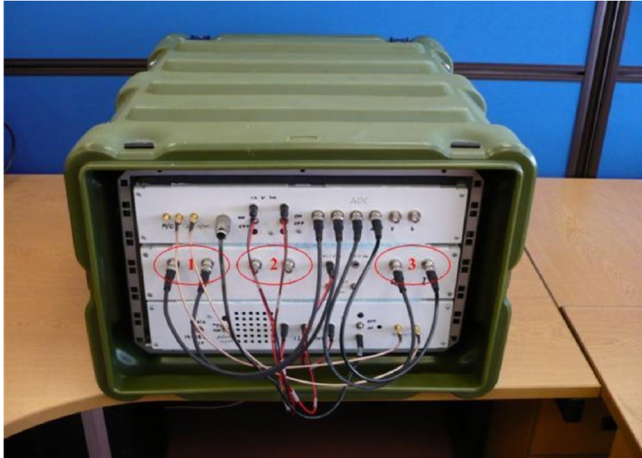
Figure 2-8: Photograph of receiver from outside
