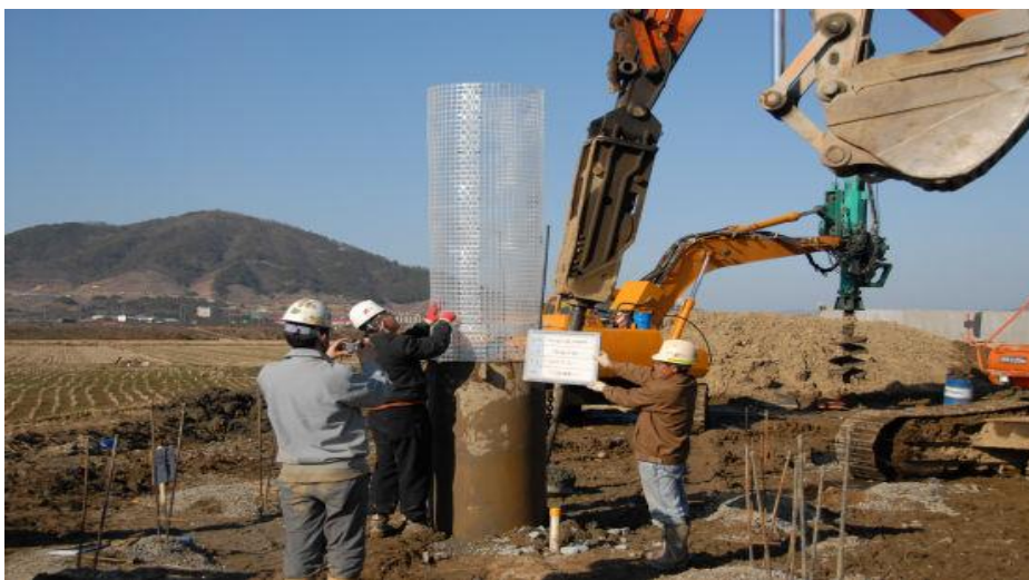
Figure 2.9: Inserting a geogrid net into a pre-bored and partially constructed stone column (Lee et al., 2008)
