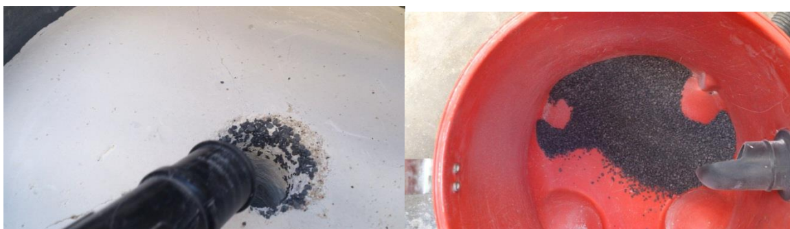
Figure 4.15: Left: Vacuuming aggregate from the stone column hole; Right: collecting the vacuumed aggregate in the storage container
