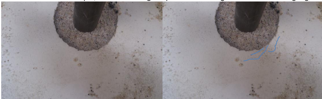
Figure 6.17: Very fine cracks around the foundation resting on the OSC, on left the original photo and on right the cracks are highlighted
