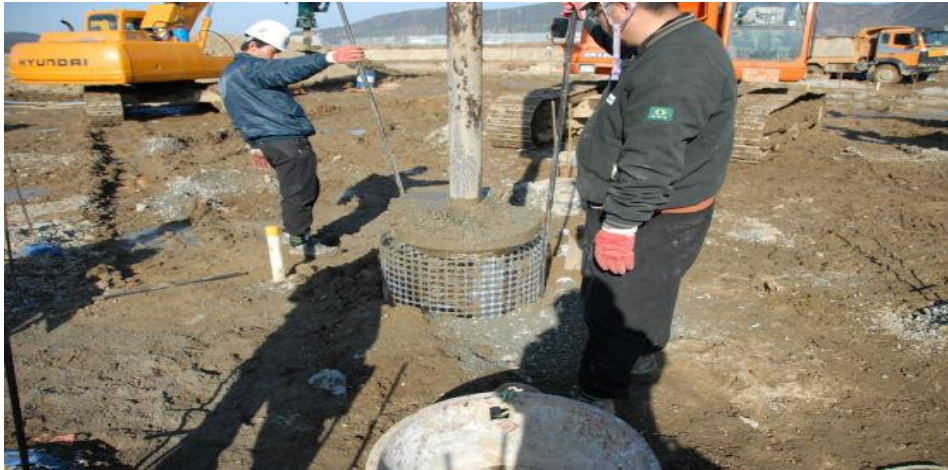
Figure 2.10: Construction of a partially encased stone column in soil (Lee et al., 2008)
