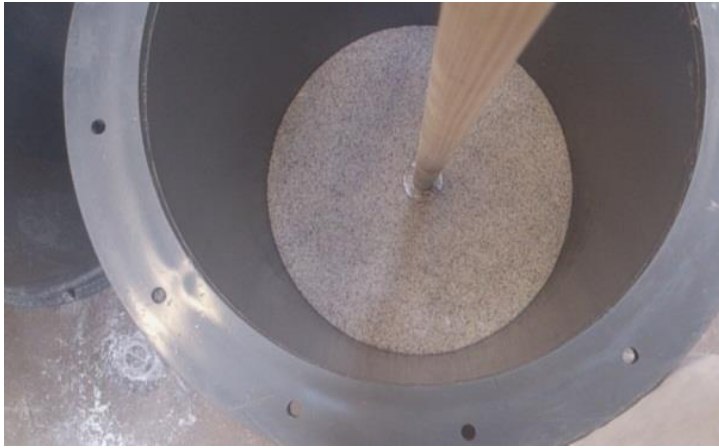
Figure 4.6: Compaction of the sand layer on top of a gravel layer, using a wooden rod
