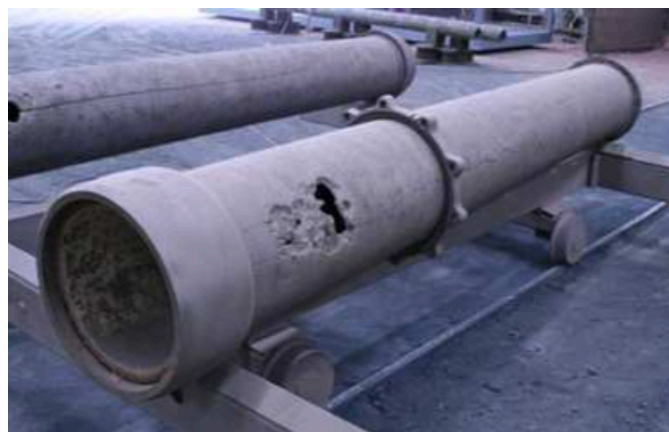
Figure 2.4 Corrosion caused by difference in the properties of the soil in contact with a pipe (Petersen, 2012)
