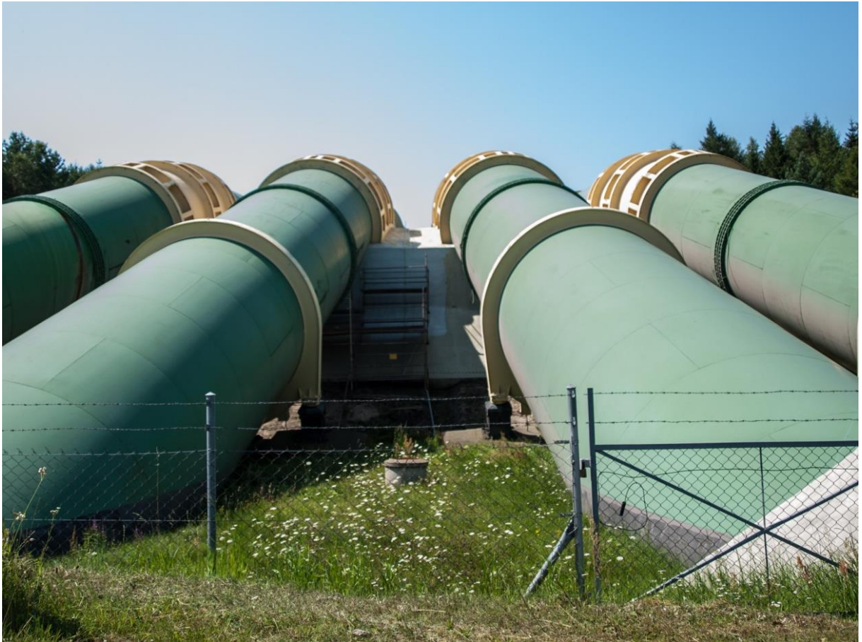
Figure 4.18 (marked ‘H’ in figure 4.1) Pipes leading up the hillside to the artificial reservoir of Żarnowiec Hydroelectric.
