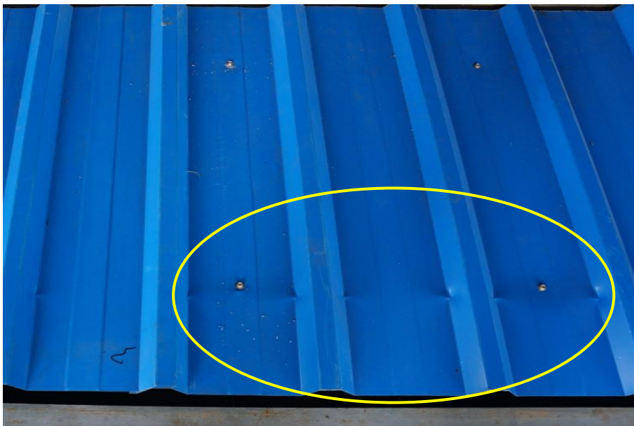
Figure 5-28: Localised deformation at the trough-crest junction
