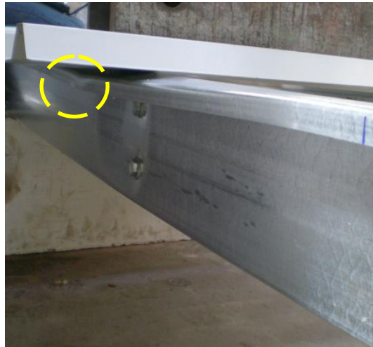
Figure 5-6: Local buckling at flange and lip
