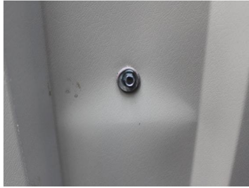
Figure 3-17: Local sheet deformation (FU)
