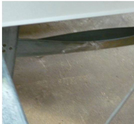
Figure 5-10: Distortion of the anti-sag bars
