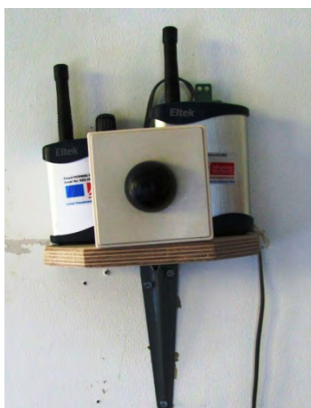
Figure 4-9: Black bulb sensor and built-in temperature and humidity sensor at 1.1m above floor level in the living space at EH
