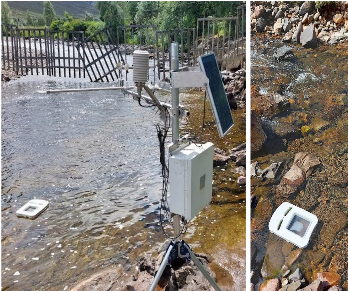
Figure 3-2 Roving AWS and floating evaporation pan installed along Clunie Water
