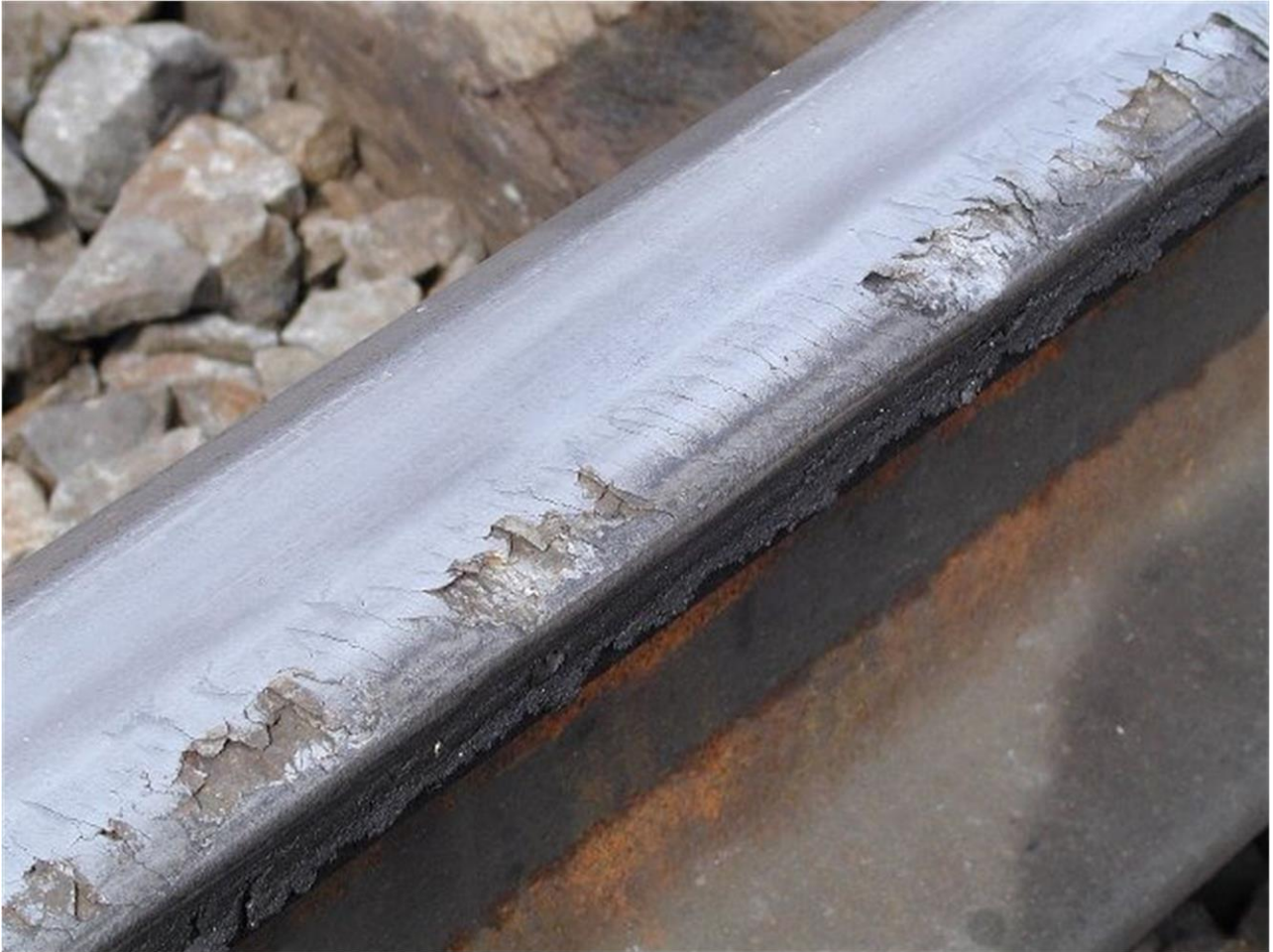
Figure 2.9 Stress corrosion on a rail [28]
