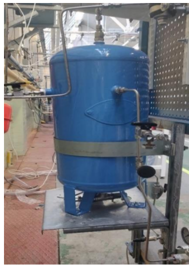
Figure 3-4 : Absorber storage tank.
