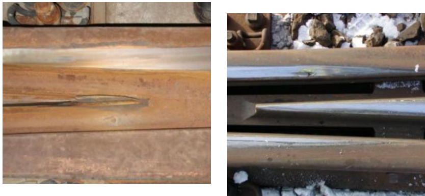
Figure 2.7 Change in shape of the crossing nose (left) and the wing rail (right) due to plastic deformation [48].
