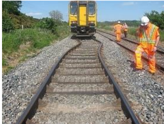
Figure 2.2 A buckled rail due to thermal expansion (Source: Skarova et al. , 2022)
