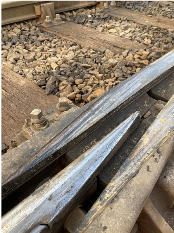
Figure 1.3 Image showing wear damage to a cast manganese crossing clearly showing a change in rail head geometry.
