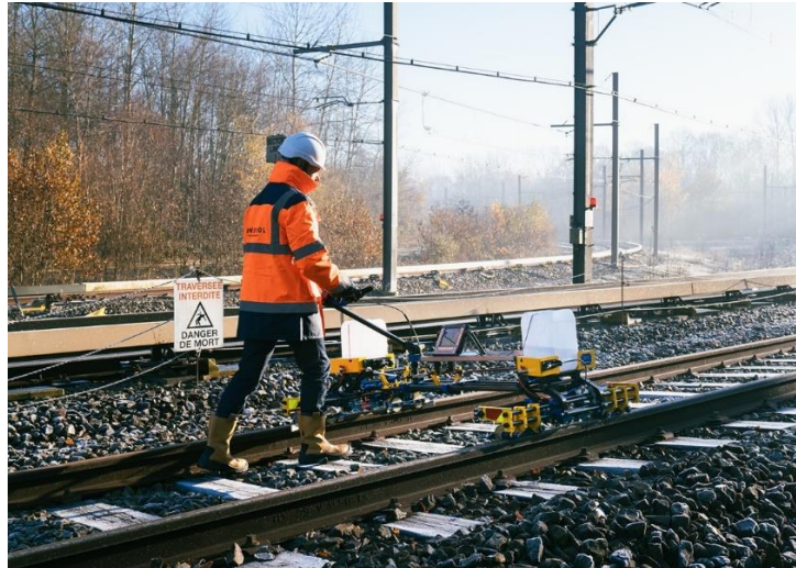
Figure 1.8 Track maintenance operative investigating the structural health of a rail section using ultra sonic techniques (Ultrasonic Rail Testing - Pandrol, 2022).
