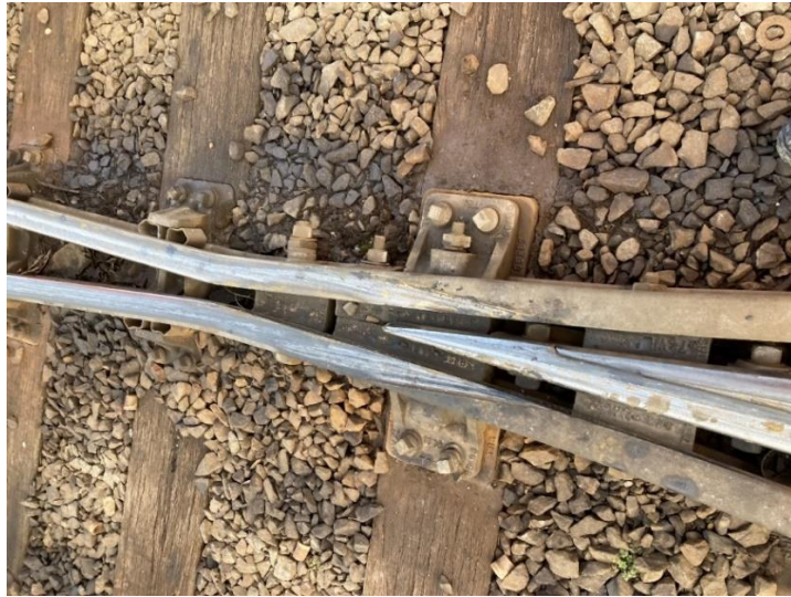
Figure 2.1 In service cast manganese crossing showing high levels of wear
