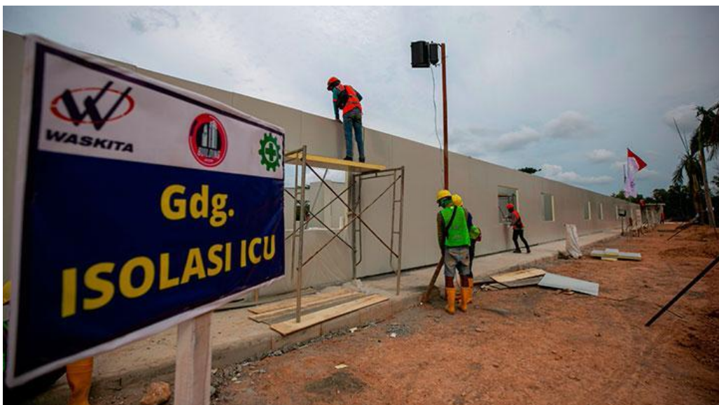
Figure 6-7. The construction of an emergency isolation hospital in Galang Camp (Source: Sahputra, 2020)
