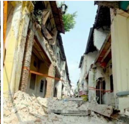
Figure 30 Collapsed of two shophouses' facade in Concubine Lane on 7/9/2011. Source: IpohEcho, 2011.
